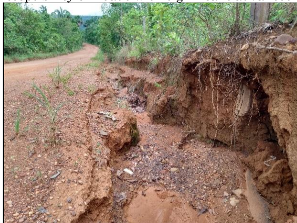
Figure 11 – High susceptibility on roads with significant advances in erosion processes.
