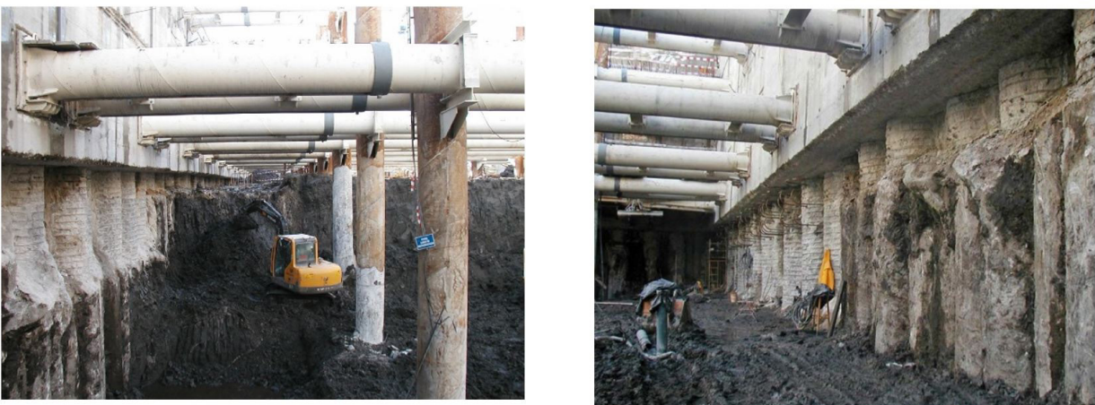
Figure 16. Excavation phase below the 3 rd struts level on the south and north walls (Brito & Fernandes, 2006a).
