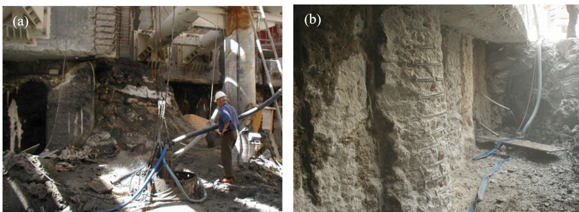
Figure 22. (a) Plug of sand bags, cement and concrete bags, about 3 m high; (b) Retaining piles from the narrow area on the north side between axes 3 and 5 after excavation up to the level -20.00 m, plug of sand bags and the underside of the lining wall at the level -18.20 m.
