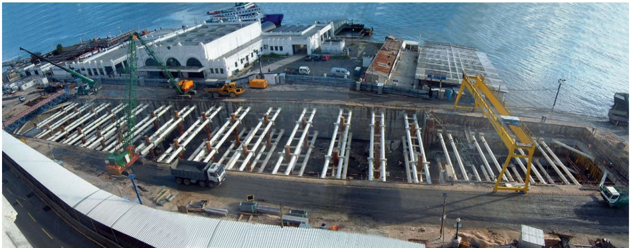
Figure 15. View of the curtain and shoring system from the Terreiro do Paço east tower (Brito et al., 2016).
