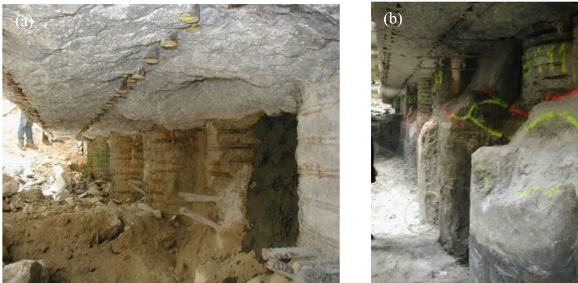
Figure 25. (a) Curtain piles at the level of the bottom slab; (b) Very significant spacing between primary bentonite-cement piles, in the foreground, and secondary reinforced concrete piles, in the background.
