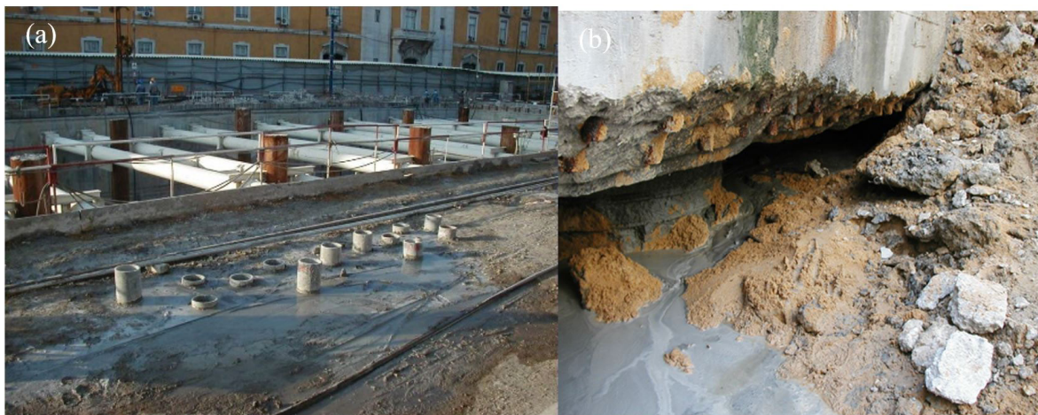
Figure 28. (a) Implantation of three rows of injection holes in the south wall in the vicinity of axis 9; (b) Injection cement grout from the outside of the curtain affluent to the interior near the corner 5 south.
