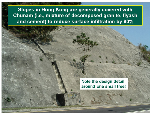
Figure 9. Use of chunam in Hong Kong to maintain the stability of slopes.
