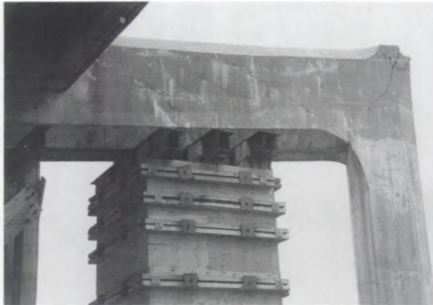
Figure 2: Cap beam flexural-shear failure (Priestley et al., 1996).
