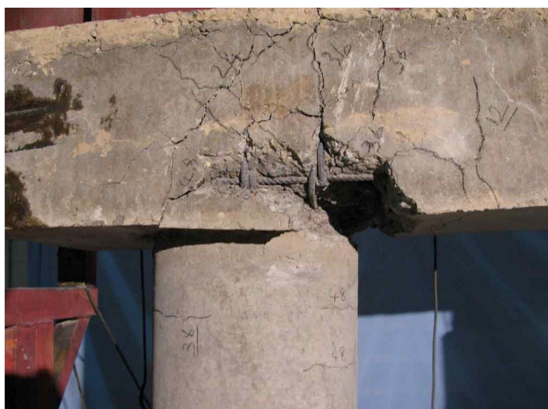
Figure 14: Spalling of the external column cap beam at relative displacement of 5.3.
