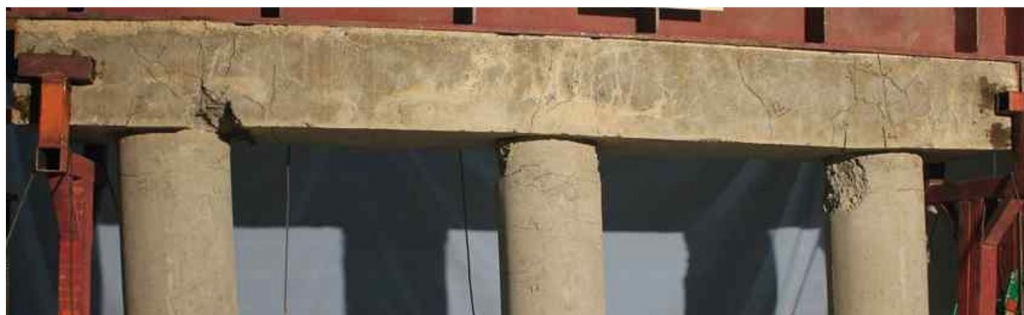
Figure 12: Damage modes in specimen A, spalling of concrete in side cap beam and middle and right column and rotation of column at relative displacement of 4.1.
